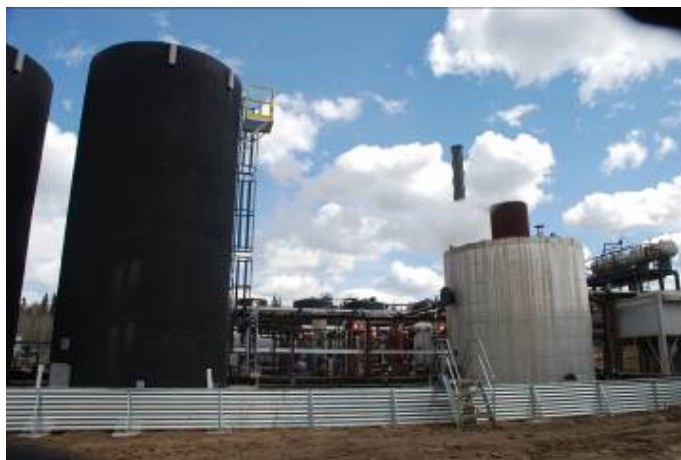
Startup of first steam at our SAGD Steam Plant Facility – May 2014.
