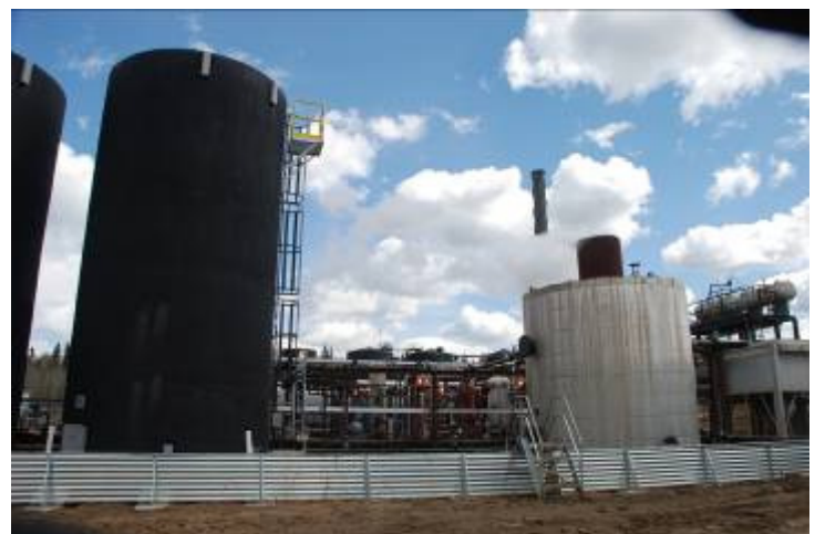
SAGD Steam Plant Facility May 2014 – Startup of first steam.
